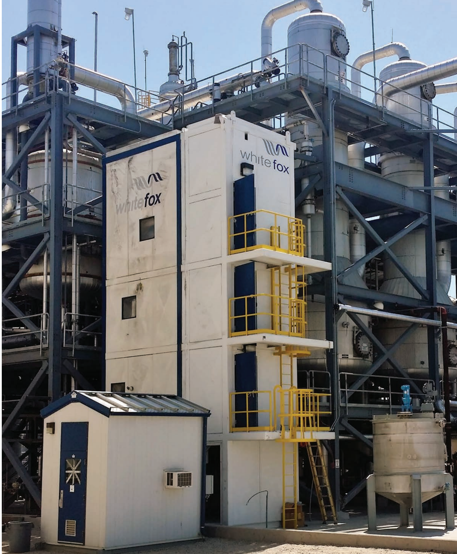
INDUSTRIAL DEMONSTRATION: Whitefox Technologies' membrane distillation is being tested at Pacific Ethanol's plant in Madera, California. Delivered flat on a semi-trailer, it was set up alongside the distillation and will be treating a portion of the regen stream from the molecular sieves, reducing energy load and addressing a cooling water limitation.
