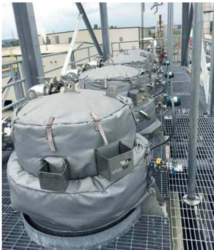
Whitefox ICE™ installed at Southwest Iowa Renewable Energy (SIRE), September 2019
